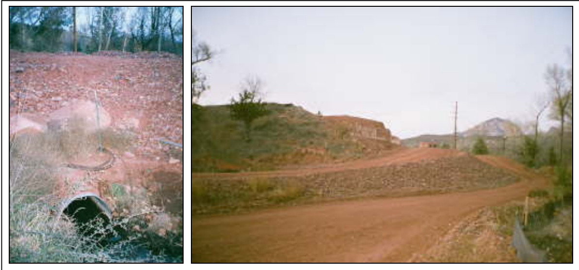
Photo 2. Red Rock Ditch showing new culvert and unauthorized fill from road construction. The ditch runs under the new road in right-hand photo
